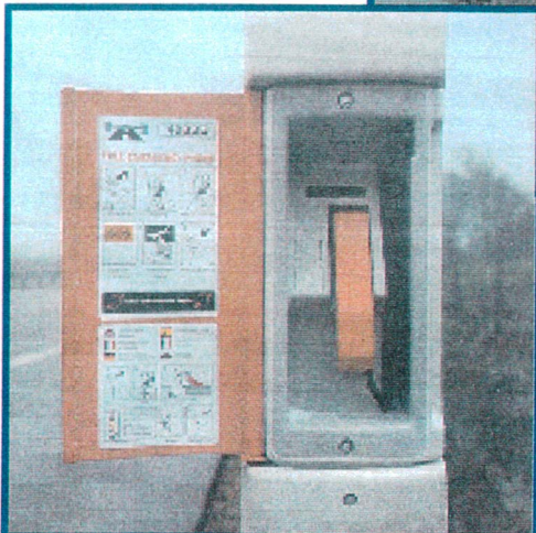
New Emergency Roadside Telephone
